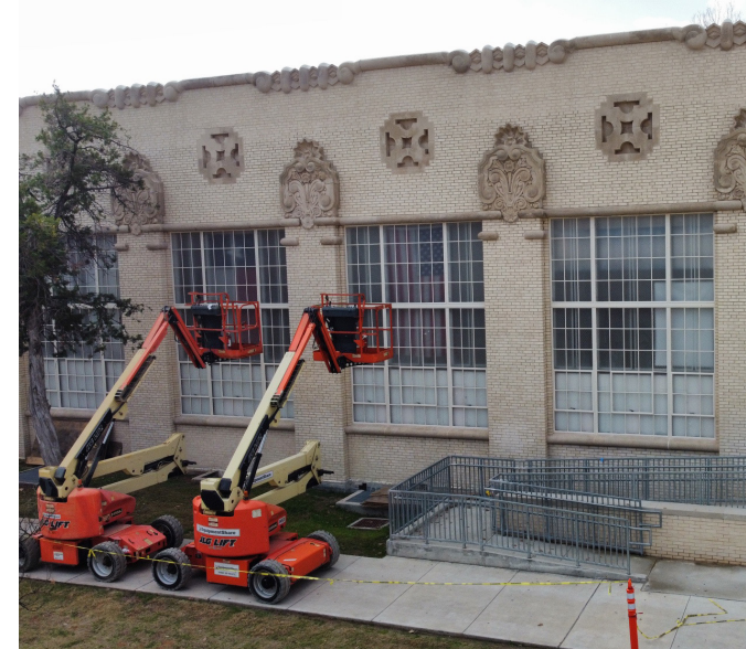
Masonry crew cleaning exterior masonry while maintained within boundaries during school operation hours.
